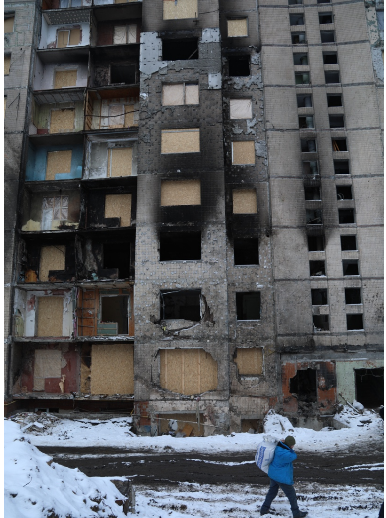
Damage to a residential building in Kyiv following a Russian air raid in September 2023. (Photo: Avedis Hadjian)
